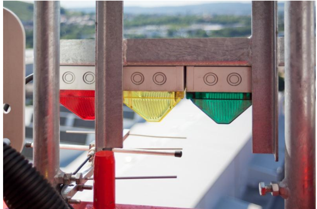
Outside light indicators showing the crane condition
