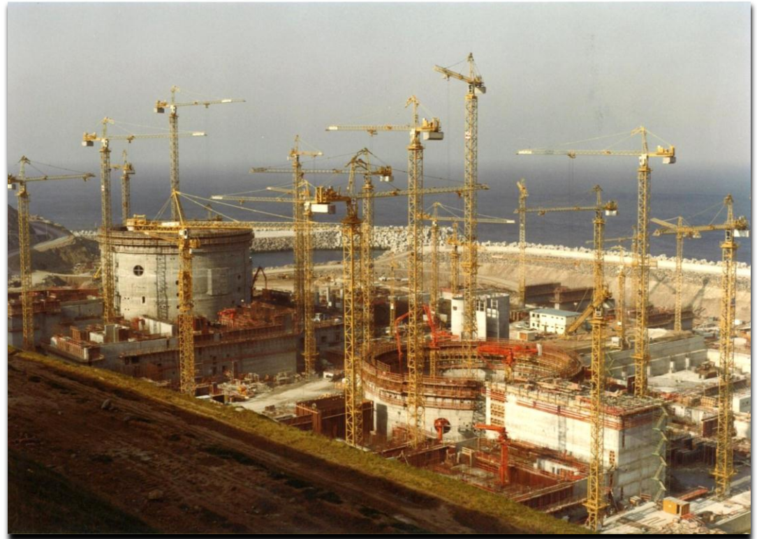
French Power Plant in the 70s
