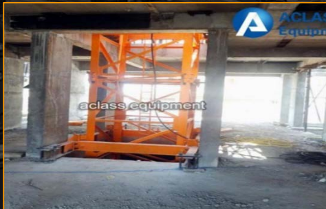
Holes/gaps in building floors
