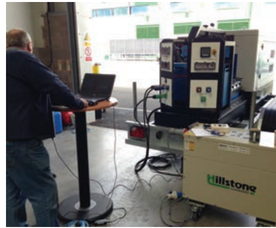
Off-Grid engineers test a lithium-ion battery system that will be used by power utility SSE.
