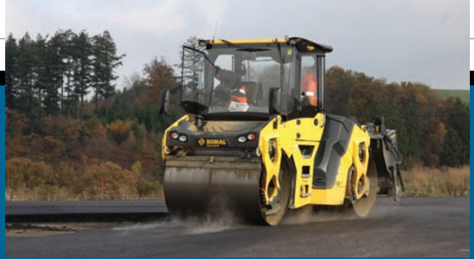
German contractor Hermann Kirchner Bauunternehmung GmbH has been using Bomag's new BW 161 ADO-5 10 t rollers featuring the company's new tangential oscillation system on a section of the B 327 'Hunsrückhöhenstraße' road connecting north Saarland and Koblenz. For the connecting sections and for processing longitudinal joints, it is usual to roll first in static mode and subsequently with vibration. With the BW 161 the tangential oscillation in the rear drum generated horizontally directed shearing forces, allowing gentle and efficient joint compaction without the need for vibration in colder weather. Bomag reports that the operators appreciated the system; "When I activate the 'TanGO', I only hear a quiet hum. It's amazing that despite this everything is so well compacted".
