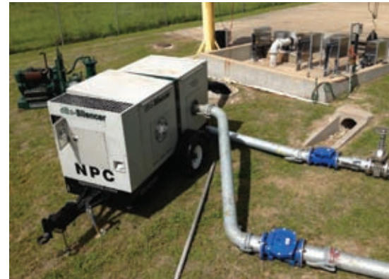
Almost 70% of National Pumps' business is with customers in oil and gas and petrochemical plants.
